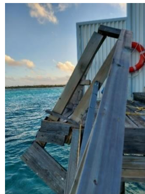
Figure 14: Damages to water bungalow
