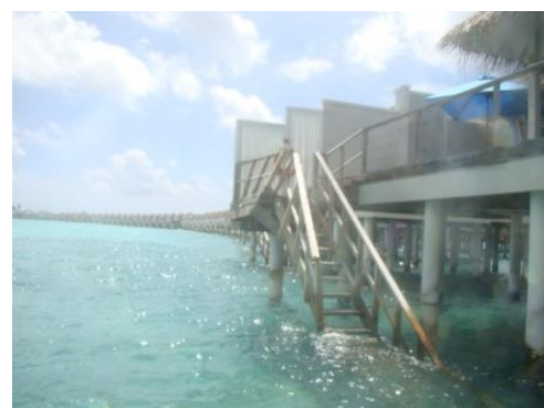
Figure 20: Damages to jetty of water bungalow
