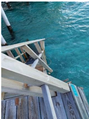
Figure 13: Damages to jetty of water bungalow
