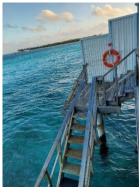
Figure 17: Damages to jetty of water bungalow
