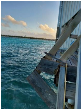
Figure 15: Damages to jetty of water bungalow
