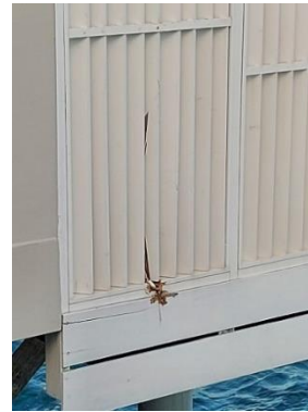
Figure 16: Damages to jetty of water bungalow
