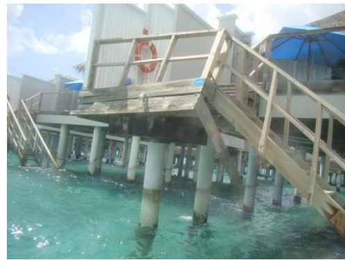
Figure 18: Damages to jetty of water bungalow
